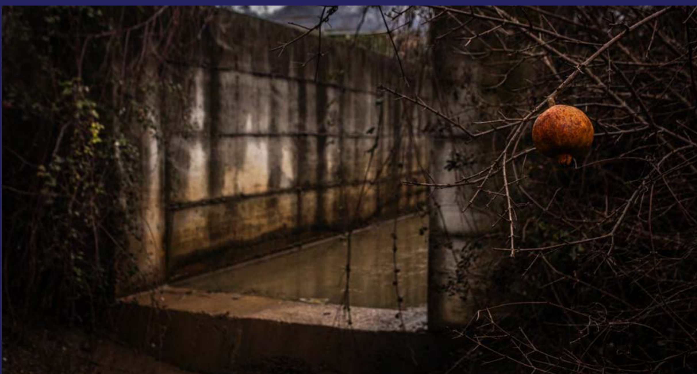
The King of Poisons leaking from the Mostar landfill (2021)
